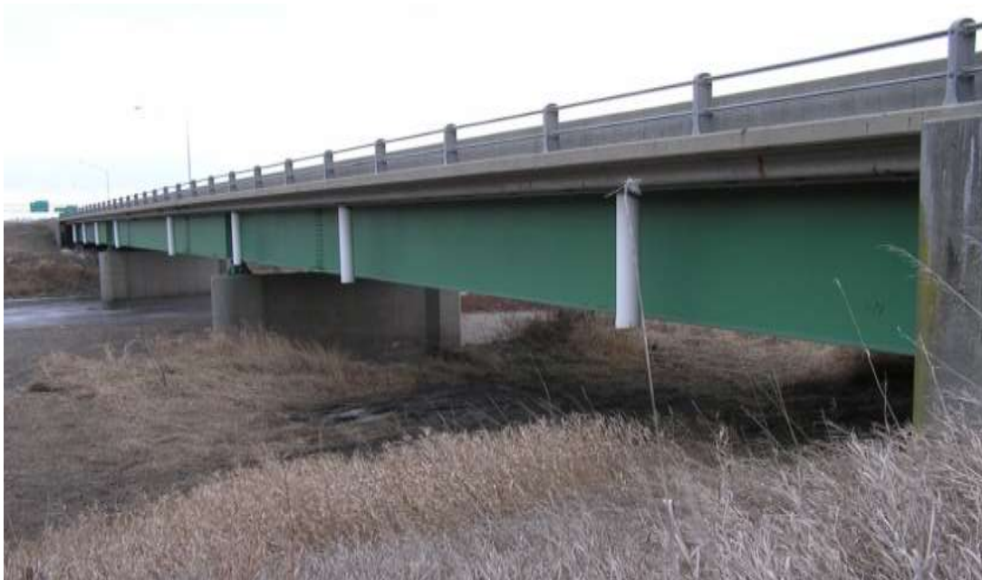
Fig. 4: Photograph of the fracture-critical Highway 30 bridge over the Skunk River near Ames, IA.
